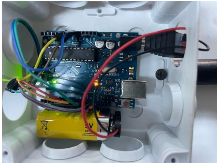
Figure 4. The Arduino control system.
